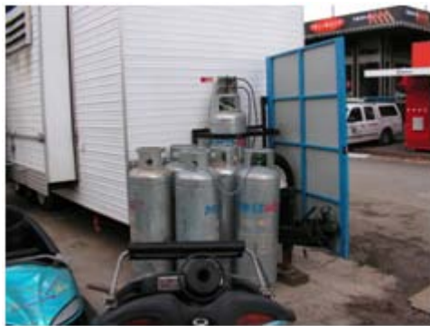
Secured to other cylinders
