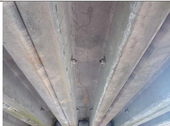
Photo 4: Cracking of u-slab beams.
