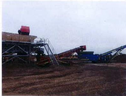
Rock Crushing Plant
