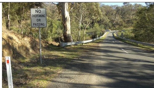
Photo 2: Looking west along Meredith-Steiglitz Road towards Coopers Bridge over the Moorabool River.
