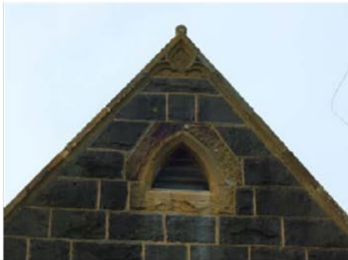
Detail of gable end showing Italian-pointed ventilator and stylised half-trefoil motif near the apex.
