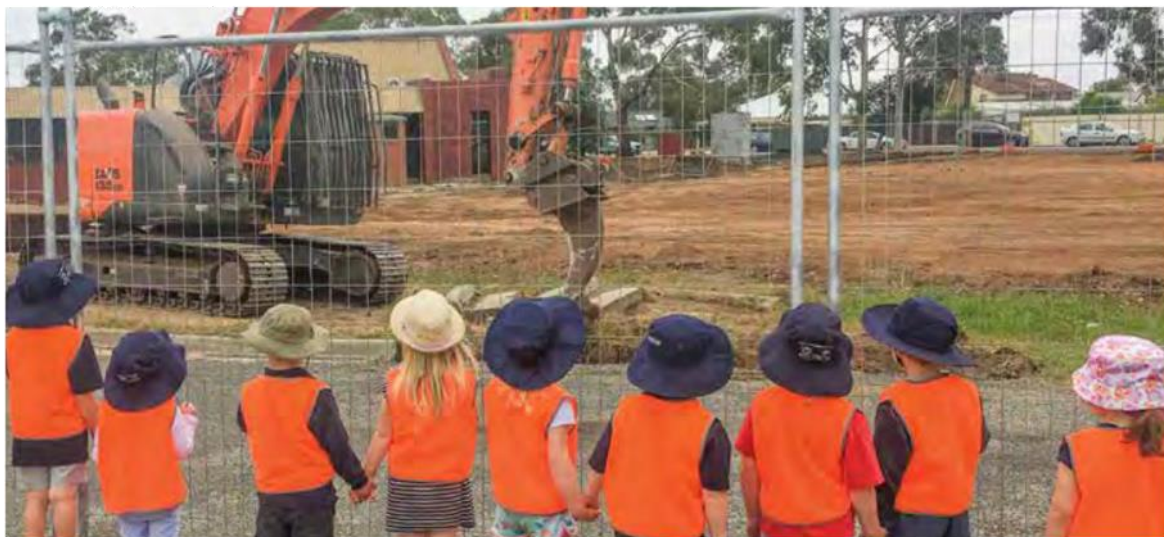
Kindergarten children from Bannockburn Children’s Service Centre watching on as construction got underway in April 2019 on the Golden Plains Civic and Community Centre.
